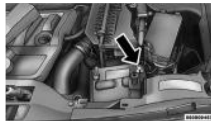
Positive Battery Post
